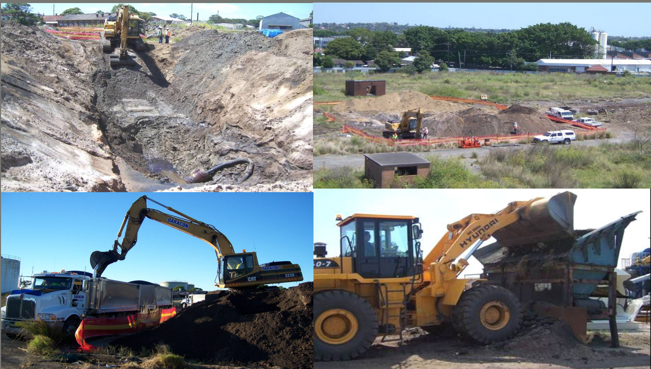
Clyde St Trial: Earthworks – excavation of 500T PAH impacted sandy soil, loading and transport of soil under license and screening of soils prior to DFTD processing.
